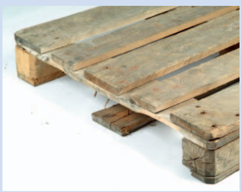
A block is missing or split to the point where more than one nail shank is visible.
