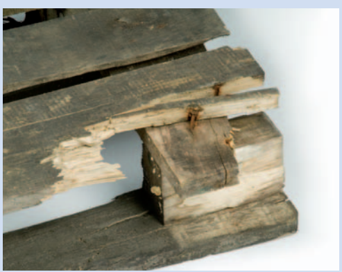
More than two upper or lower leading boards are damaged and reveal one nail or screw shank for each board.
